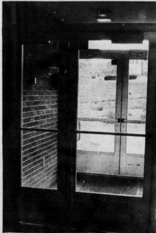
These new doors, designed to permit easier accessibility for wheelchairs to and from classroom buildings, were part of the SRSC renovation. The renovations will add to the new SRUP statue. (Photo by Kimbo.)
